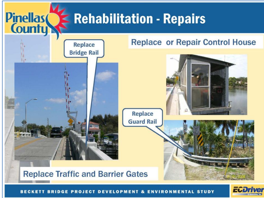
Figure 3.5– Rehabilitation Repairs – Replacement of Guard Rail, Bridge Rail, Traffic and Barrier Gates, and Control House
