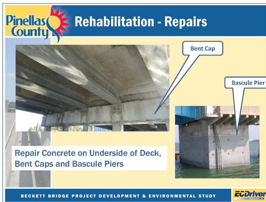
Figure 3.8 – Rehabilitation Repairs – Concrete Repairs to Underside of Deck, Bent Caps, and Bascule Piers
