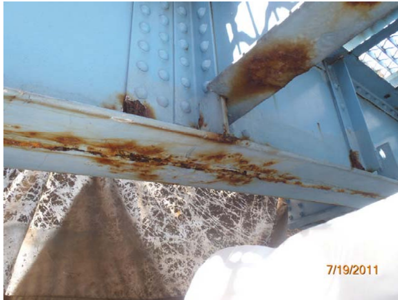
PHOTO 9: 152/4 Paint Stl Floor Beam
