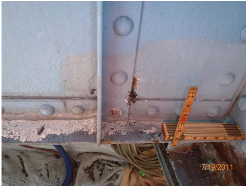
PHOTO 10: 152/4 Paint Stl Floor Beam
