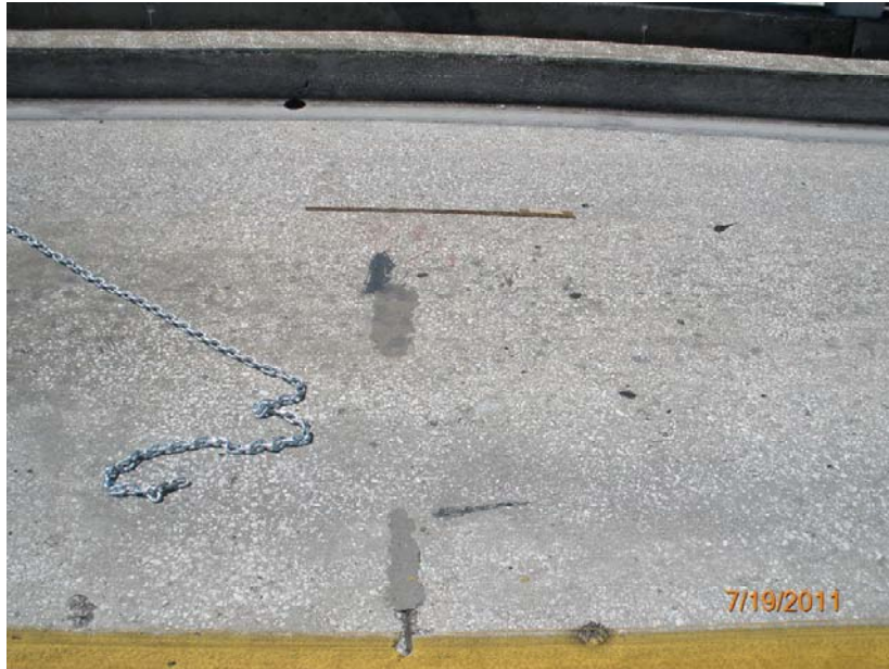
PHOTO 33: 12/4 Bare Concrete Deck
