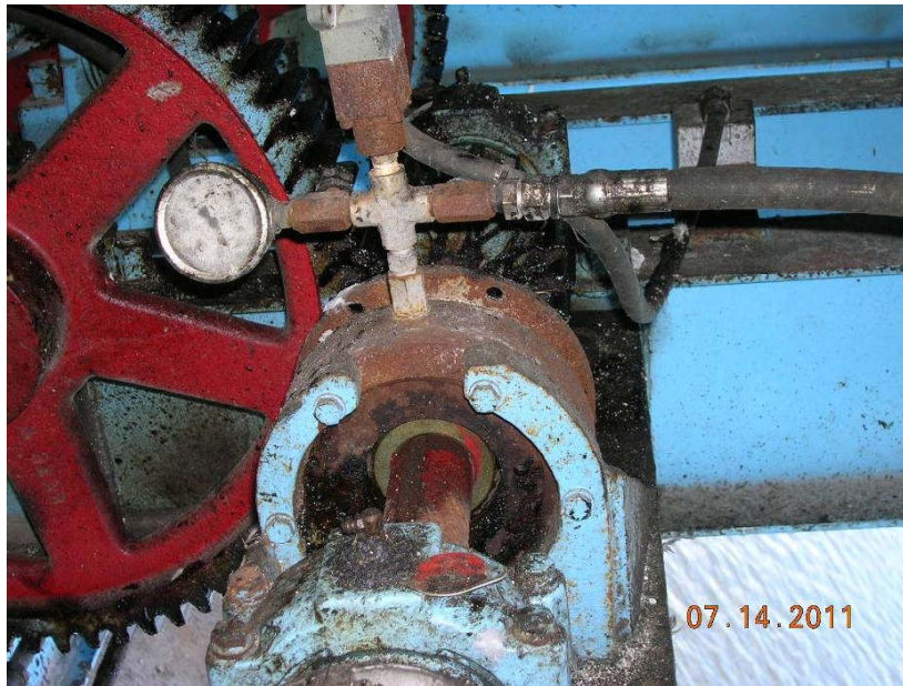
PHOTO 12: 544/4 Brakes & 548/4 Hydraulic Piping Sys
