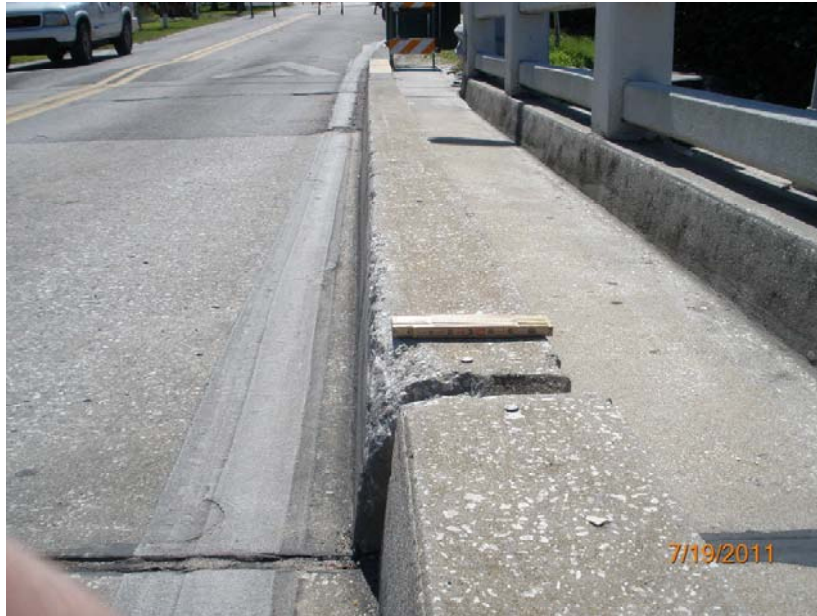
PHOTO 31: 12/4 Bare Concrete Deck
