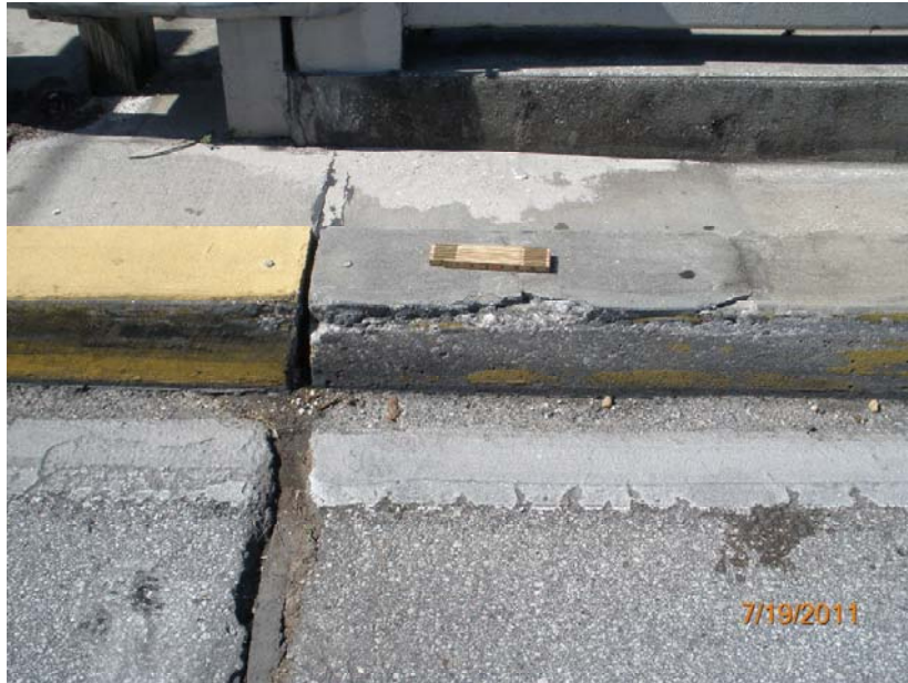
PHOTO 34: 12/4 Bare Concrete Deck
