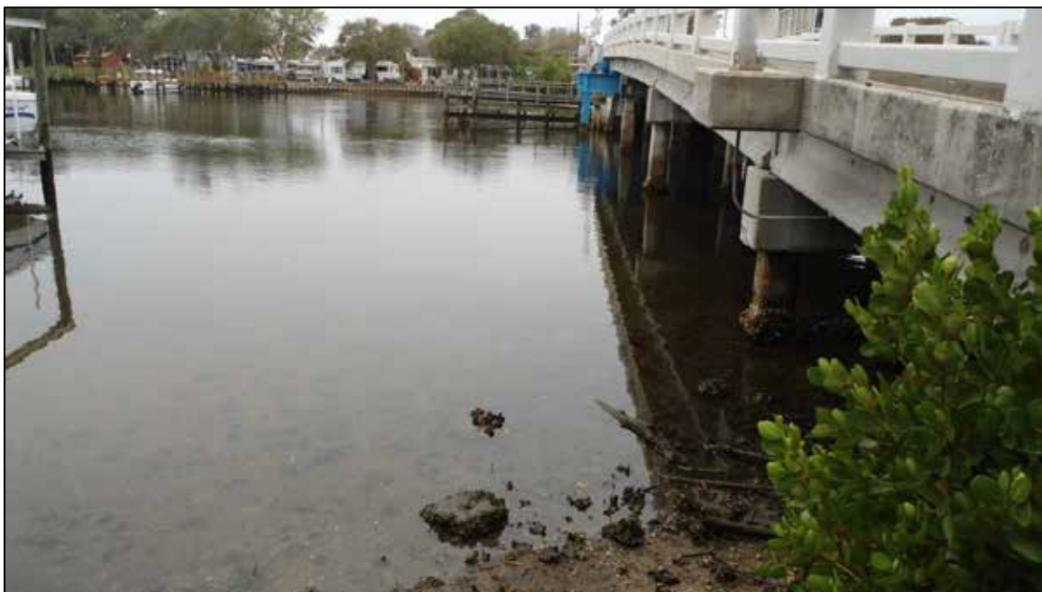
Photo 6: East side of Whitcomb Bayou on the south side of Beckett Bridge, facing west.
