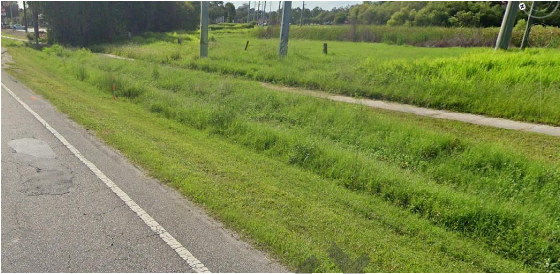
10. OSW-11 a drainage ditch, facing southeast located along Gibsonton Drive.
