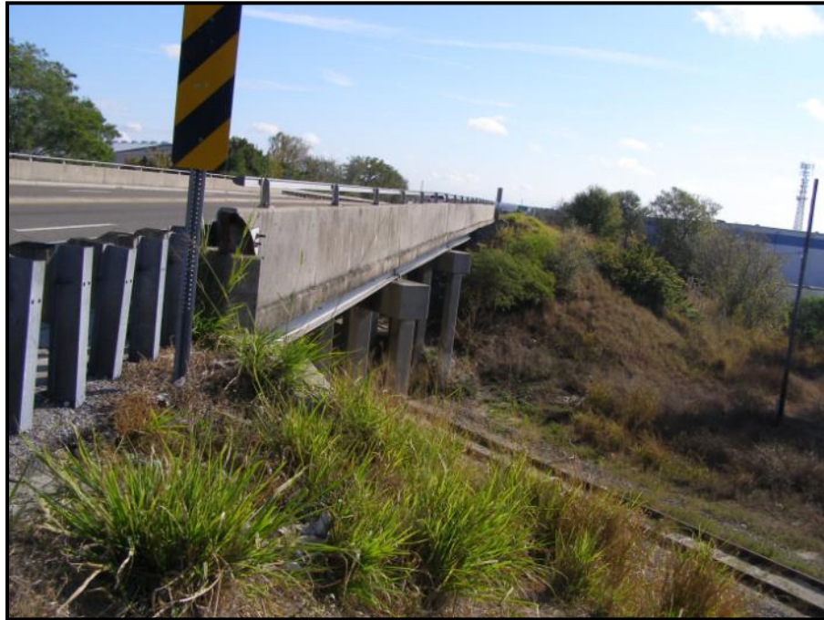
Photo 5.12. South elevation of the SR 600/US 92/Hillsborough Avenue over CSX Railroad Bridge (FDOT No. 100021), 8HI11687.
