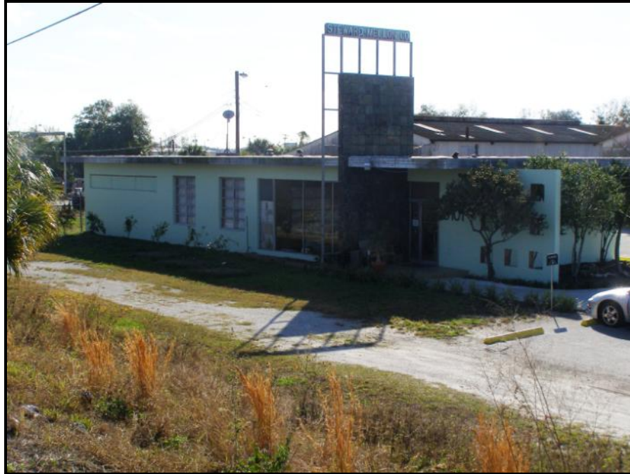
Photo 5.6. North and west elevations of Building 1 (8HI11669) of the Steward-Mellon Company Resource Group (8HI11684) at 5101 East Hillsborough Avenue.
