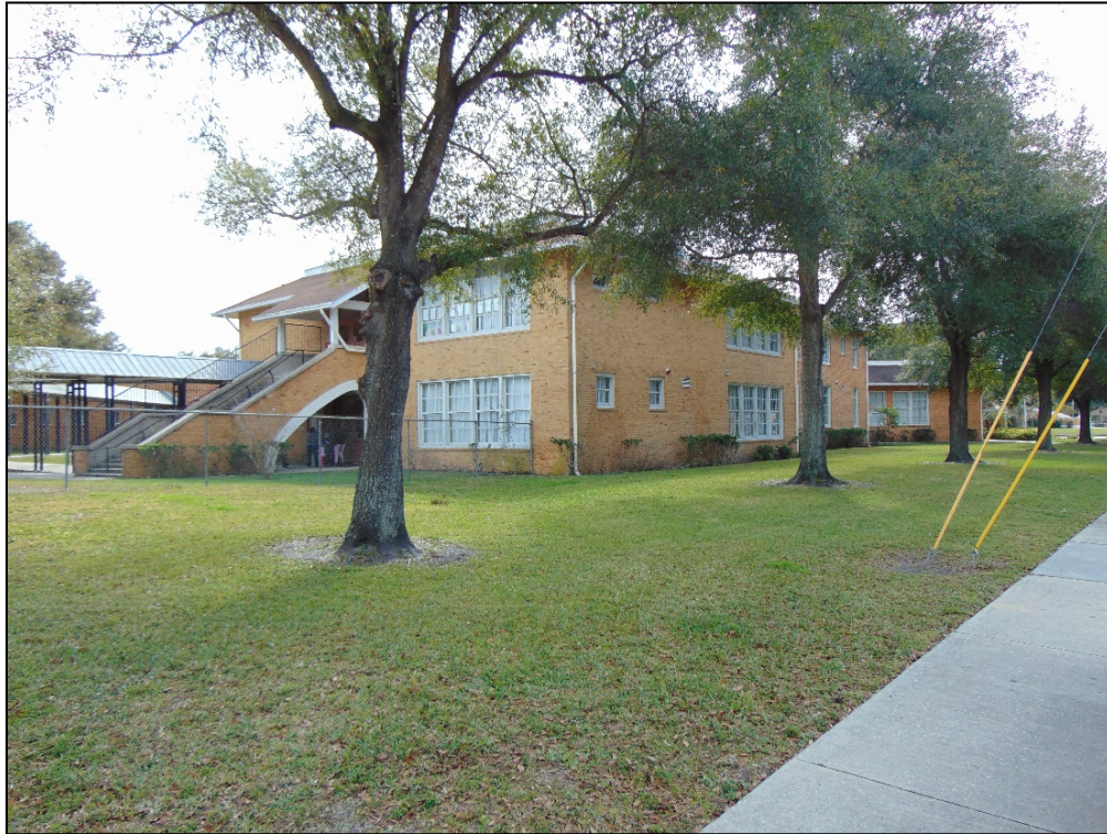
Figure 41: The Concrete Exterior Stairs of the North Wing of Seminole Heights Elementary School/6201 N Central Avenue (8HI12539), facing Southwest
