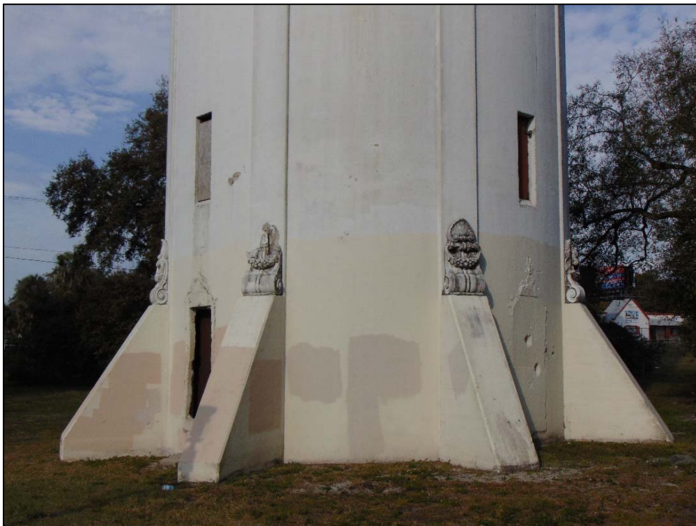
Figure 59: The Concrete Buttresses of the Water Tower with Foliated Shell Motif Embellishment, facing Northwest
