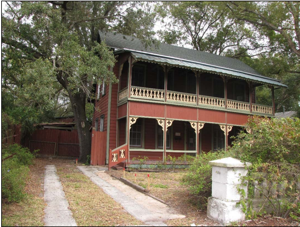
Figure 56: National Register–listed Captain William Parker Jackson House/800 E Lambricht Street (8HI11581), facing North
