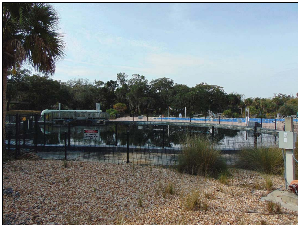
Figure 17: A Photograph of the Contributing Concrete Retaining Wall Pool within the Sulphur Springs Park Resource Group, currently closed, facing Southwest
