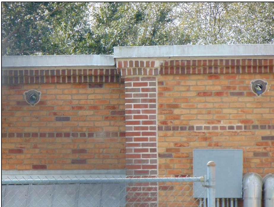
Figure 3: Polychromy and Pilasters of Seminole Heights Elementary School/6201 N Central Avenue (8HI12539), facing south
