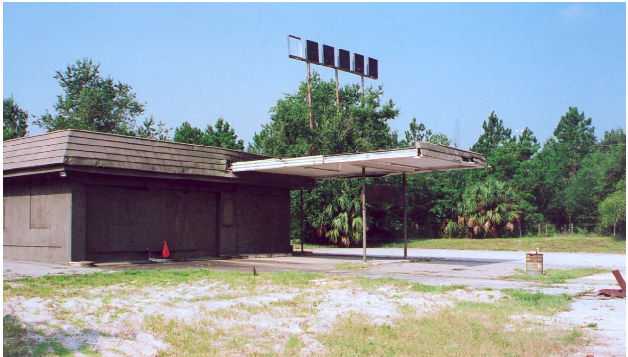
Site #3- view looking southwest toward former Texaco #203-132. Note open hatch covers on bottom right.
