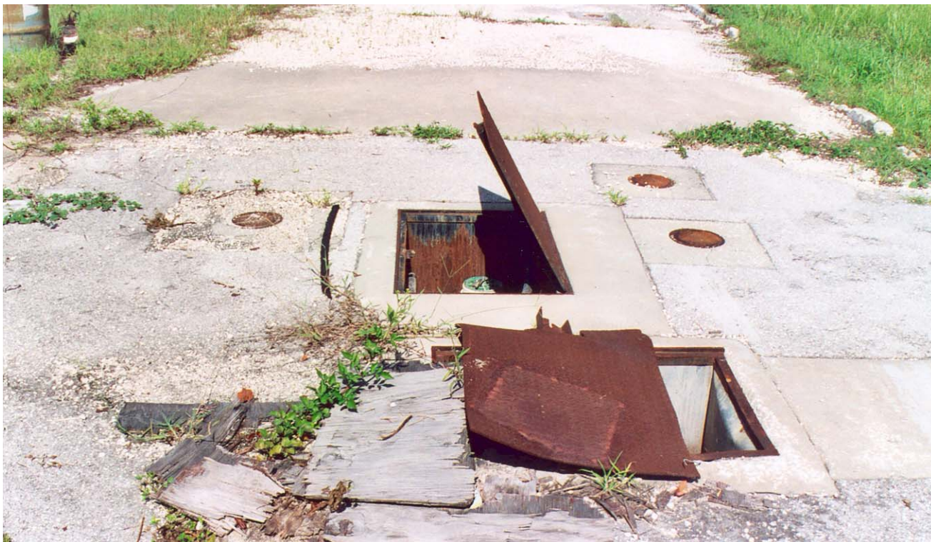
Site #3- closer view of open hatch covers possibly reveals evidence of suspected tampering at former Texaco #203-132.
