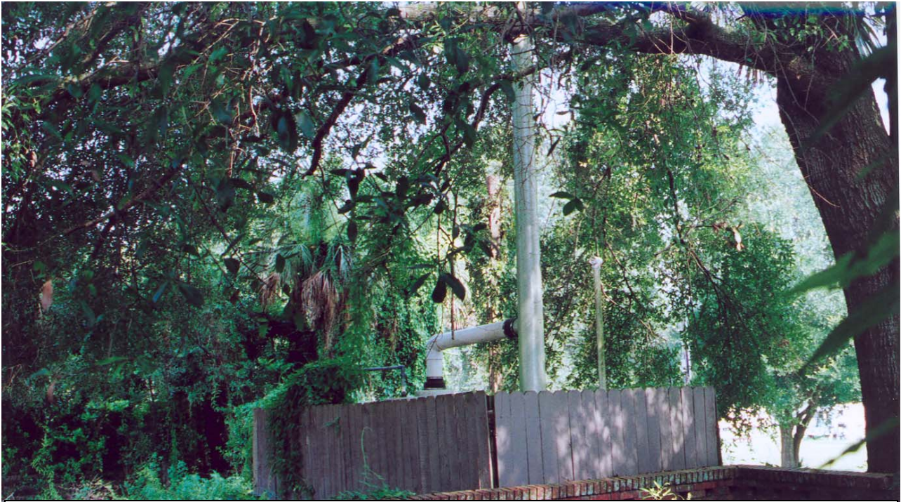
Site #2- view of air stripper located on western side of building at the former Exxon #5285 on SR 50 east of I-75 ROW.
