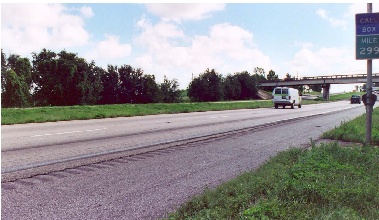
Site # 4- Near MP 299 was area of tanker spill in Jan 2004. Rated MEDIUM
