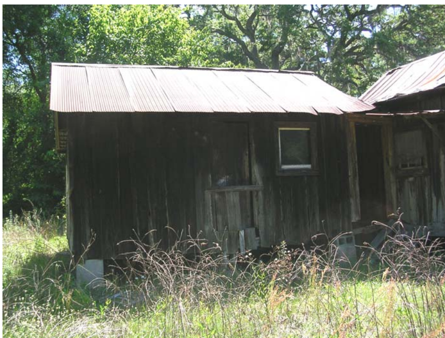
Photo 6.10. The St. Clair/O'Neal Homestead Residence (8HE554), west elevation of breezeway and kitchen house.
