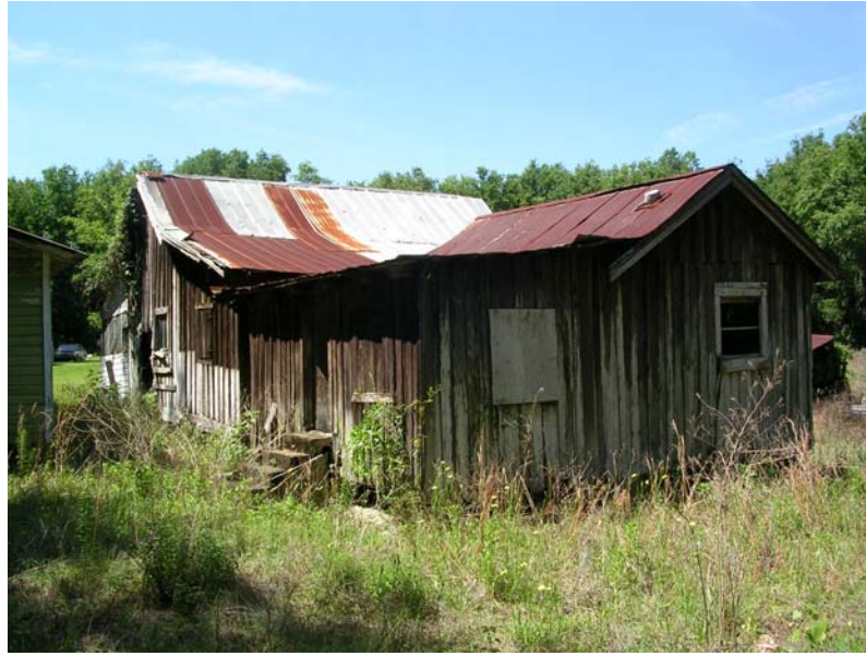
Photo 6.11. The St. Clair/O'Neal Homestead Residence (8HE554), north and east elevation of breezeway and kitchen house.
