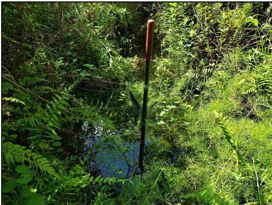
Photo 4. Standing water in SMF 21A.
