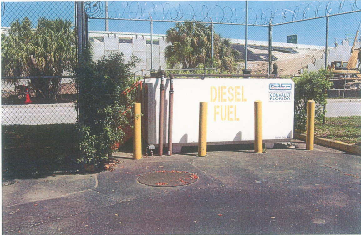
View of aboveground diesel fuel tank located on the former county jail property located on the project site.
