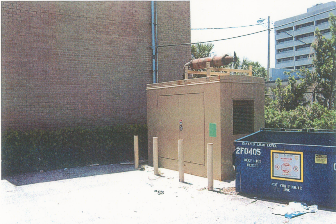
View of diesel powered emergency generator on Chem-Tel, Inc. parcel located at 1305 N. Florida Avenue (on central portion of project site).
