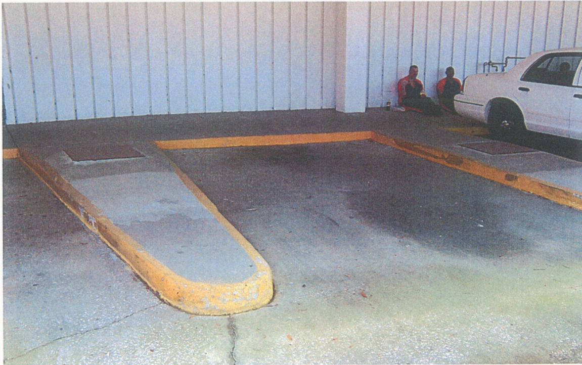
View of what appears to be UST fill ports located south of the aboveground diesel fuel tank shown above.
