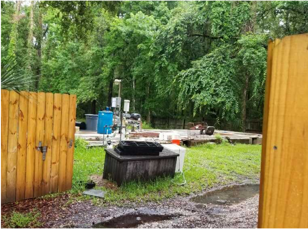
Site 11: Countryside Estates Wastewater Treatment Plant taken from Tall Oaks Lane looking south; Photo Taken June 14, 2019
