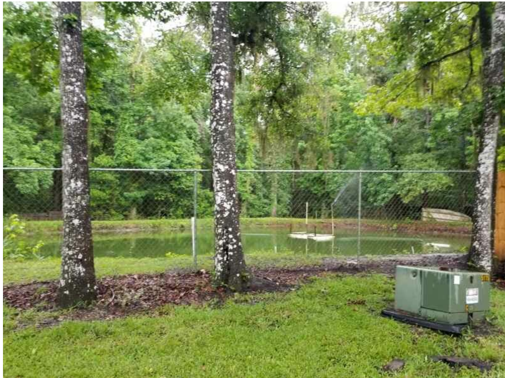
Site 11: Countryside Estates Wastewater Treatment Plant taken from Tall Oaks Lane looking east; Photo taken June 14, 2019
