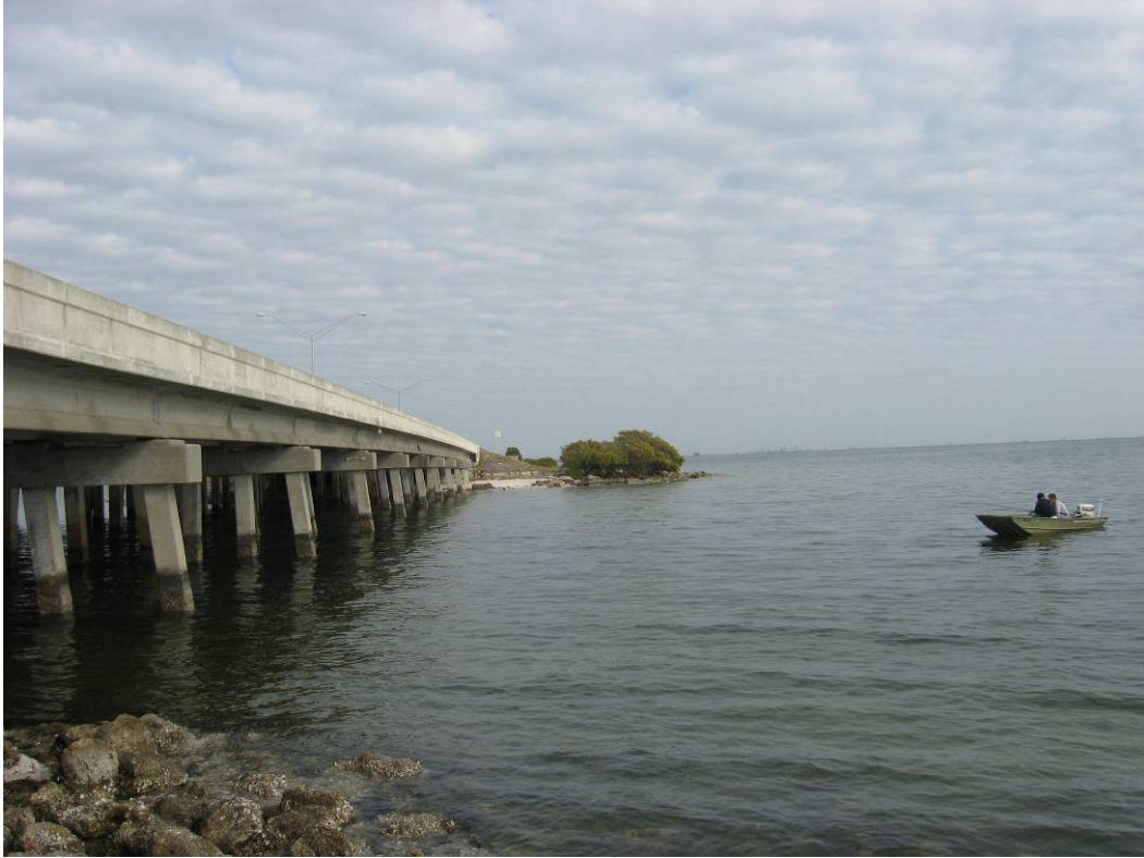
Picture 1 – South side of Causeway on west side of Structure 1 facing east
