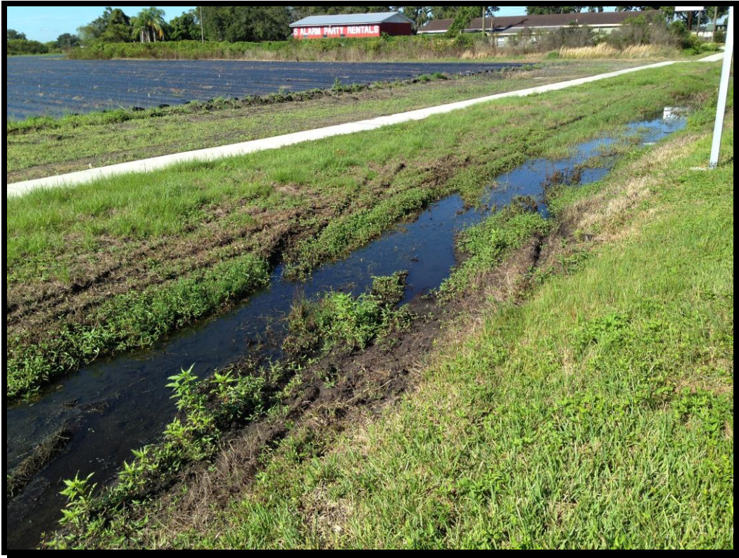
SR 60 PD&E (District 7) Representative photo facing southwest Surface Water 10S Ditch south of SR 60 (FLUCFCS – 641x /NWI PEMx)
