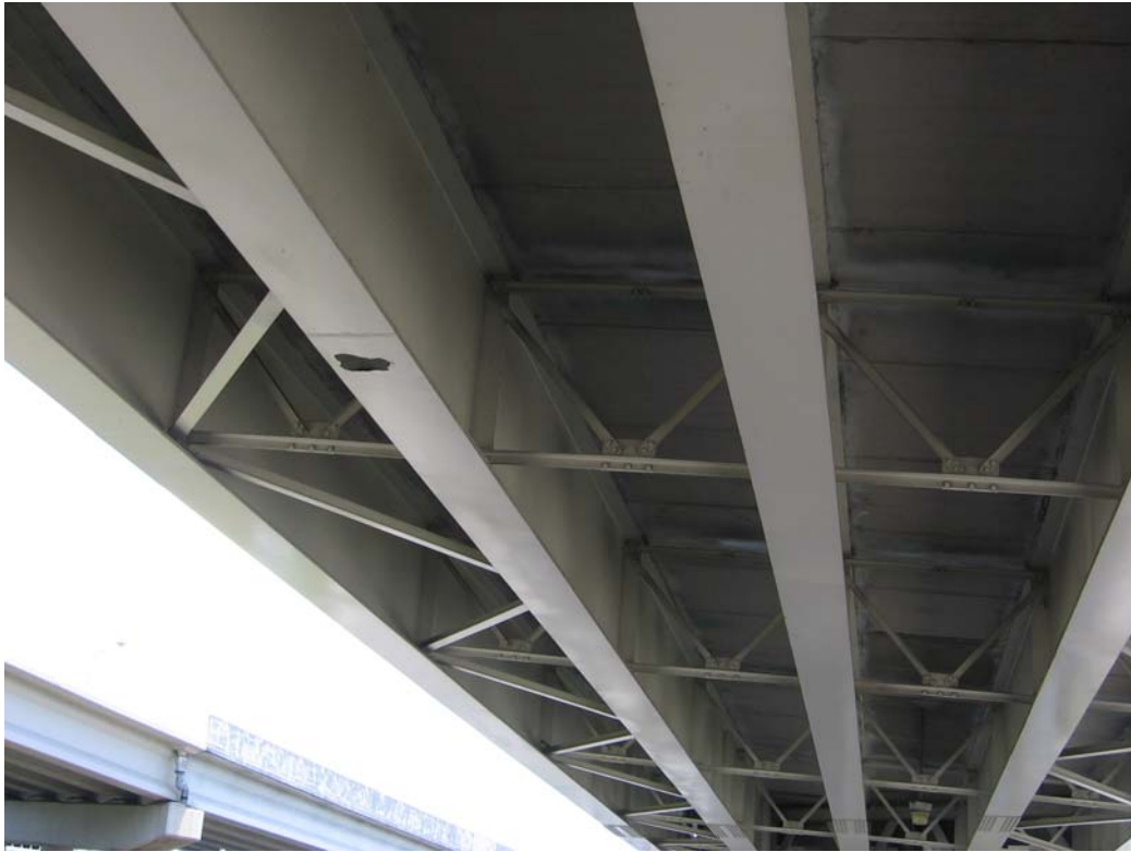
PHOTO 5 – 10/07/09 – SAMPLE RCRA-1.4 GRAY PAINT ON METAL SPAN 35
