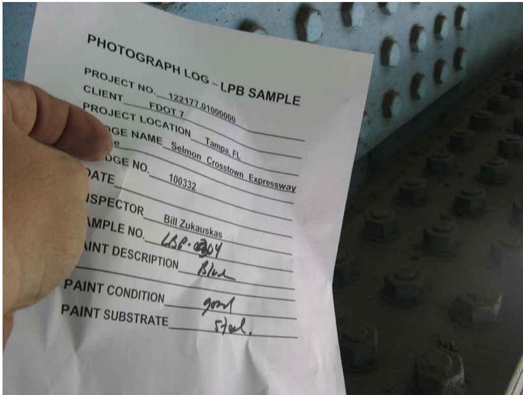
PHOTO 7 – 10/02/09 – SAMPLE RCRA-3.4 BLUE PAINT ON METAL SPAN 10 (OVER BROREIN STREET)
