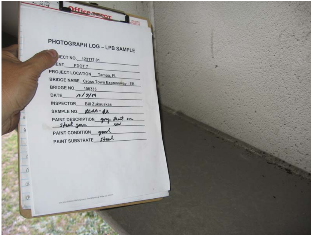
PHOTO 3 – 10/07/09 – SAMPLE RCRA-1.2 GRAY PAINT ON METAL SPAN 35
