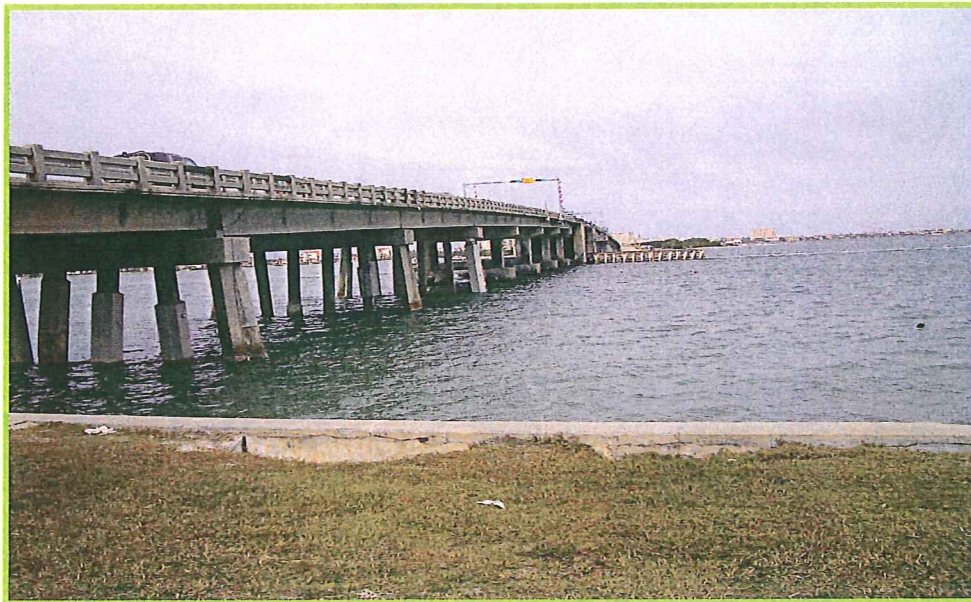
Photo 18 – View of Tierra Verde Bridge (Bridge No. 150049) – Site No. 5 – Facing north along the east side of the bridge (station 285+00)
