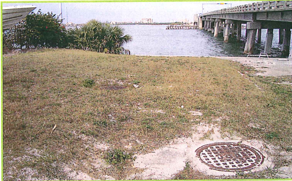
Photo 19 - View of Tierra Verde Bridge (Bridge No. 150049) – Site No. 5 – Facing north along the west side of the bridge and utilities (station 285+00)
