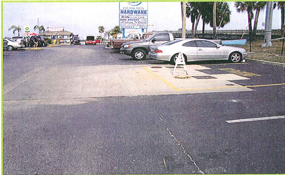
Photo 11 - View of Texaco-Tierra Verde Marina/BP Station – Site No. 4 – Close-up view of underground fuel storage tank farm located west of S.R. 679 (station 278+00)
