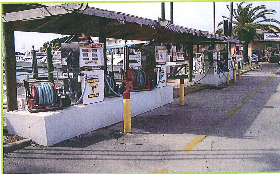
Photo 3 – View of Tierra Verde Resort & Marina – Site No. 1 – Close-up view of the dockside fuel pumps (station 268+50)
