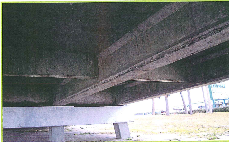
Photo 20 – View of Tierra Verde Bridge (Bridge No. 150049) – Site No. 5 – View of underside of concrete bridge (station 285+00)
