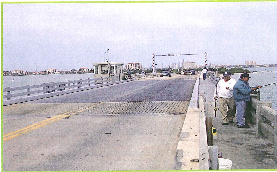
Photo 21 - View of Tierra Verde Bridge (Bridge No. 150049) – Site No. 5 – View of the steel draw bridge (station 285+00)
