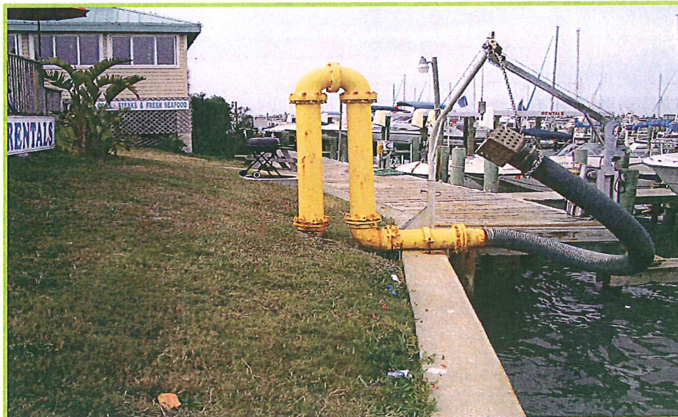
Photo 12 – View of Texaco-Tierra Verde Marina/BP Station – Site No. 4 – Close-up view of fuel lines located west of S.R. 679 (station 279+00)
