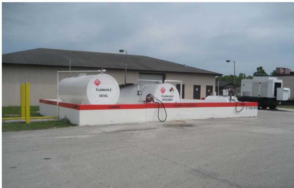
6. View to the northeast of three ASTs located at Site No. 5 - Zephyrhills Correctional Institute
