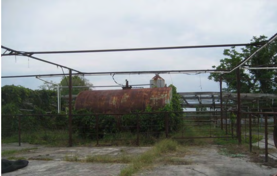
9. View to the south of the second AST located at the abandoned farm facility Site No. 6 – Neil Rucks Dairy
