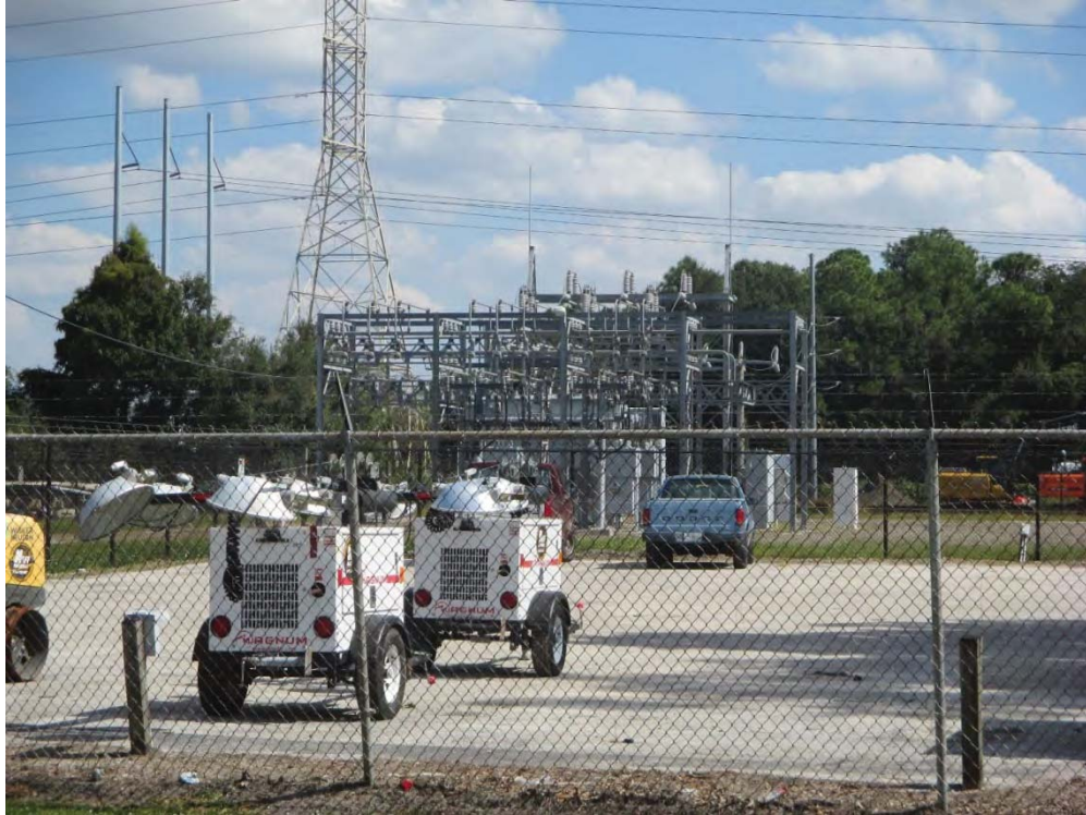
45. View to the east of Site No. 65 – Electric Substation (4343 US 301)
