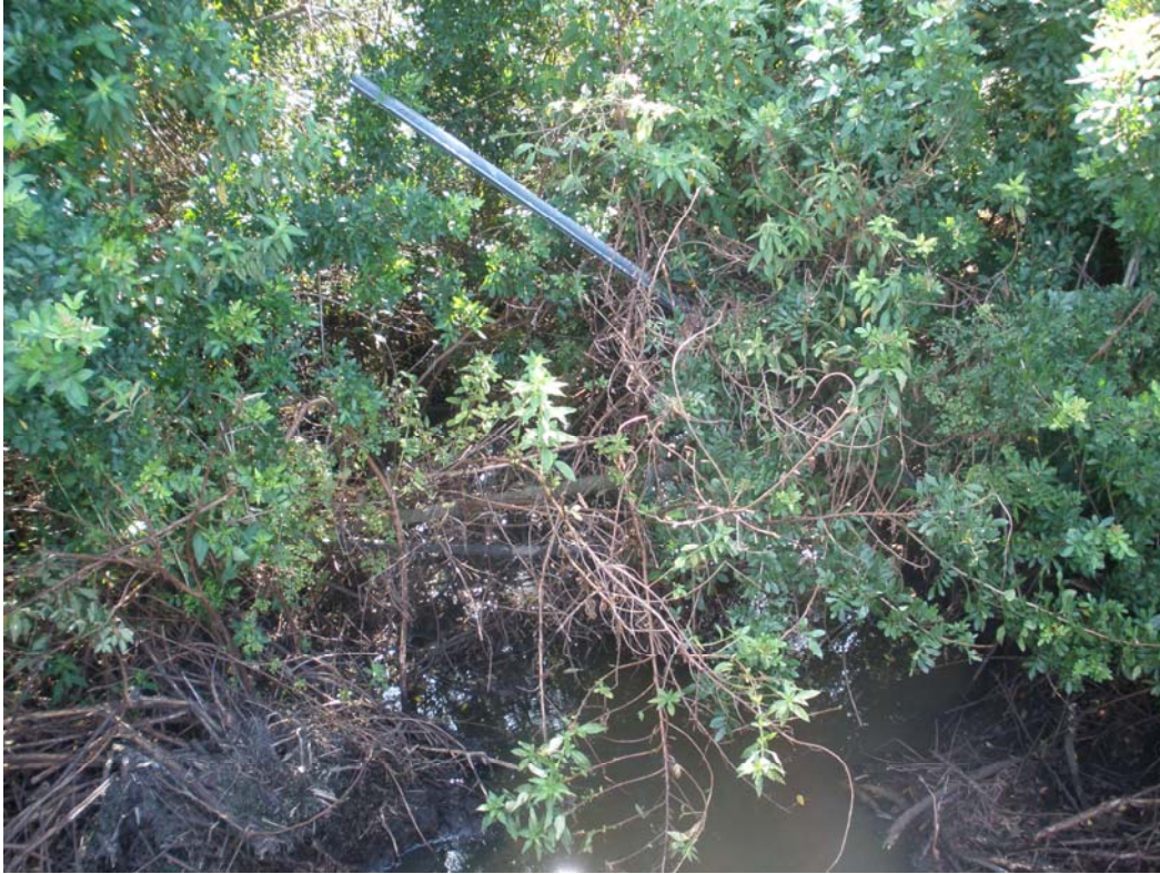
Overgrown ditch running perpendicular to roadway – 8/7/2008
