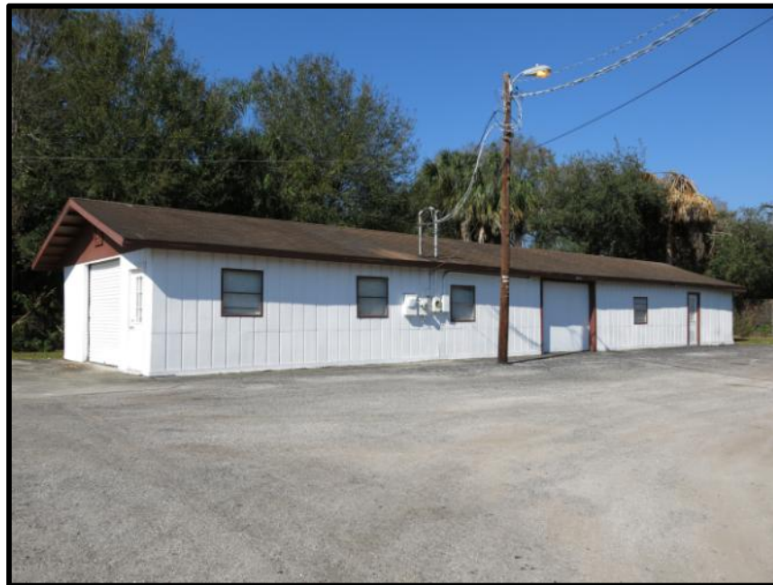
Photo 5-16: The east and south elevations of the Frame Vernacular storage building at 10829 S US 41 (8HI12078).
