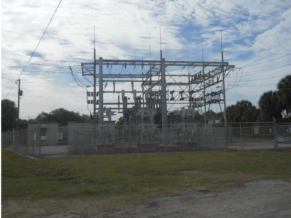
PHOTO 25 Site No. 25 - Electrical Substation Located at Sam Warren Road and Tamiami Trail.
