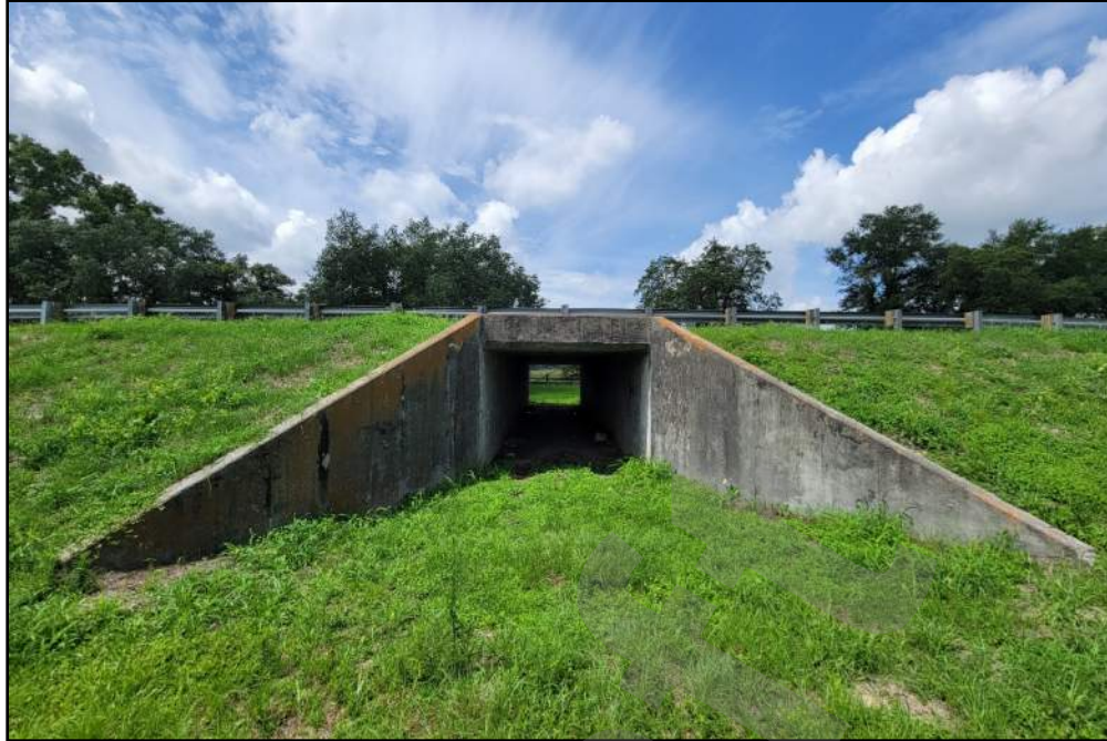
Photo 5-24 Typical example of a cattle pass box culvert within the APE. US 98 Cattle Pass #2 (8PA03349), looking southeast.
