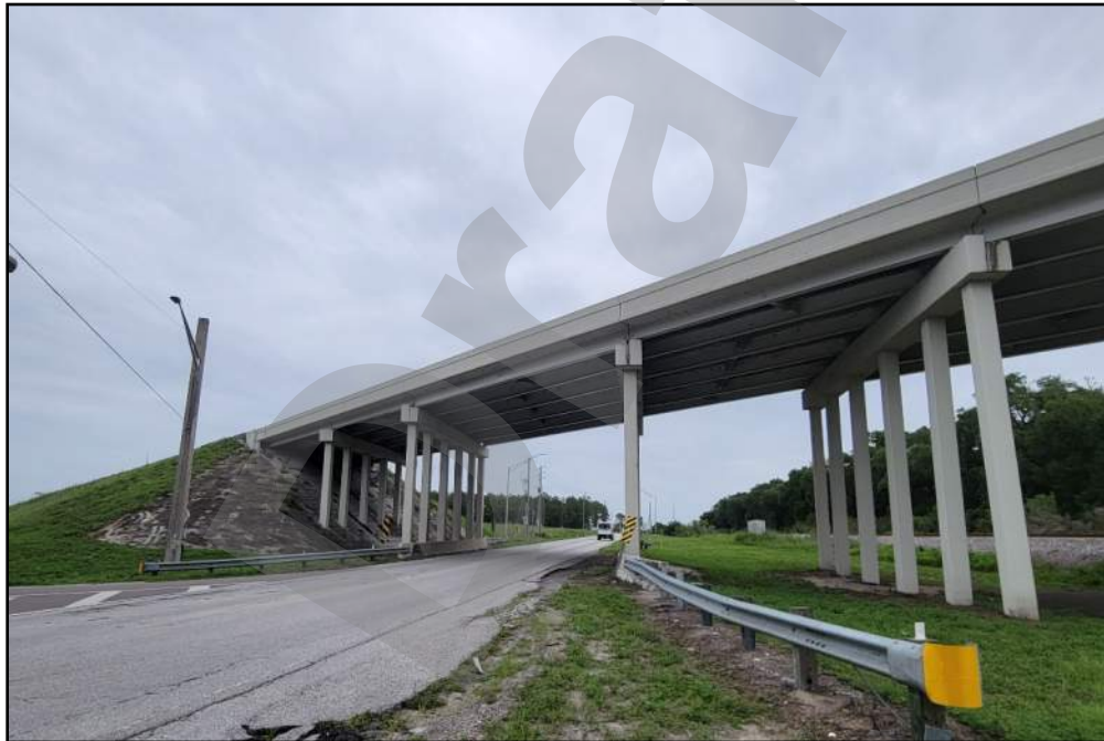
Photo 5-23 Typical example of a stringer (multi-beam) bridge within the APE. US 98 over CSX Railroad/CR-35A (Bridge No. 140025) (8PA03356), looking north from Old Lakeland Hwy/CR 35 Alt.
