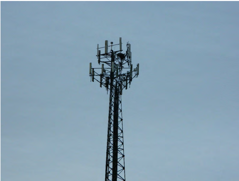
Photo 4: Nest in Cell Tower near US 98 and CR 54 Intersection
