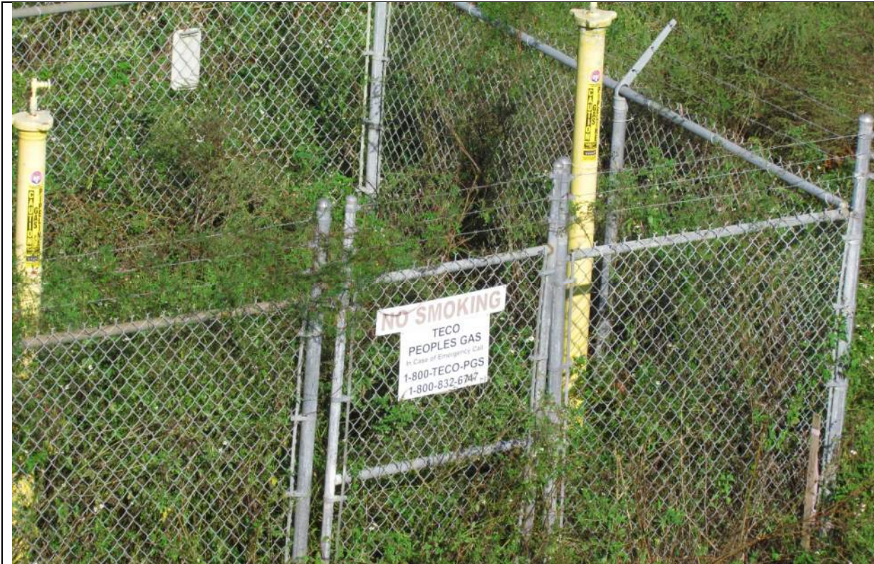
TECO Gas Utilities near CSX
