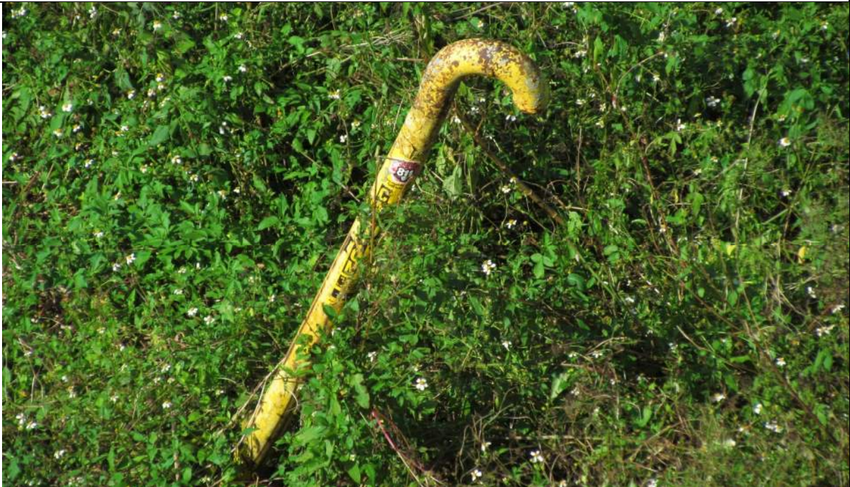
Bent Natural Gas Marker
