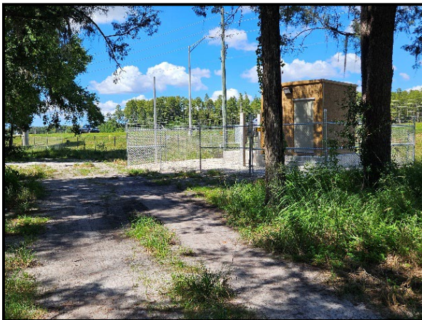
Photo 2.23. View of utility station in the northeast corner of Pond P1E1, facing north-northwest.
